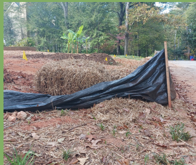
Failing or improperly installed silt fencing
